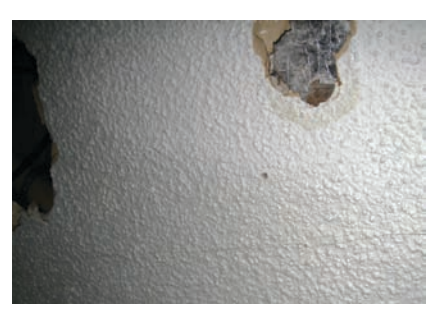
CEILING (DETAIL2) The hairline crack where water damaged the ceiling a second time.
