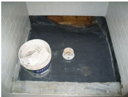
AFTER THE TILE WAS REMOVED Shows the shower pan liner with tile removed.
