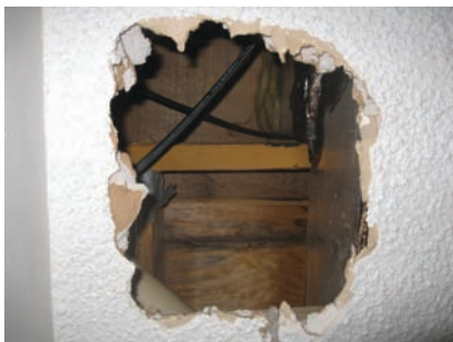
CEILING (DETAIL1) Shows the damp plywood where the water came through.
