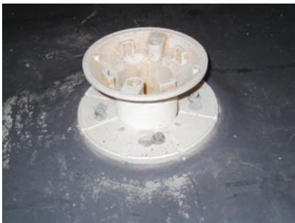
SLOPED UP TO DRAIN Shows the shower pan liner actually sloping upwards towards the drain. Water has to climb uphill to get out.
