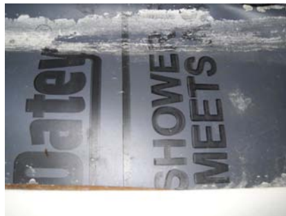
OATEY SHOWER PAN LINER 'A Bath Pro' would not install the shower pan liner according to the manufacturer's installation instructions.
