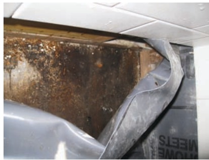
DETAIL 1 Another view showing the wet plywood directly beneath the shower pan liner. (Should be a mortar bed.)
